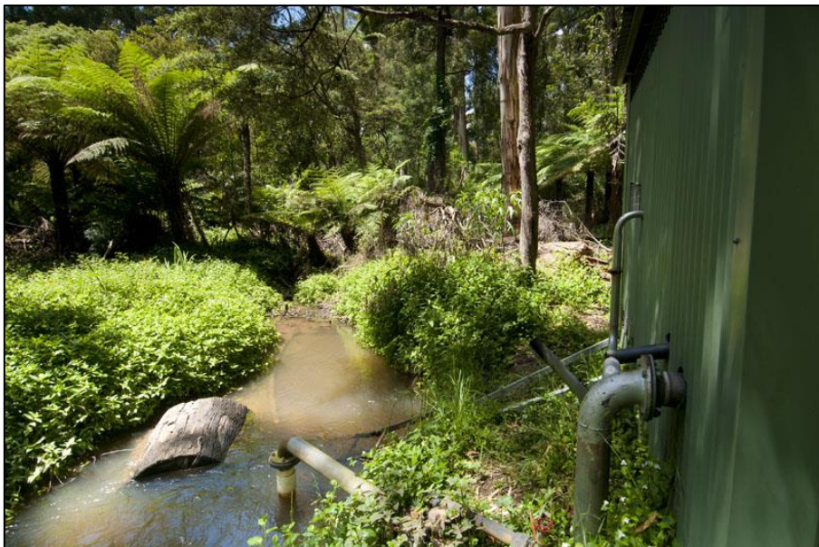
Pump on waterway
