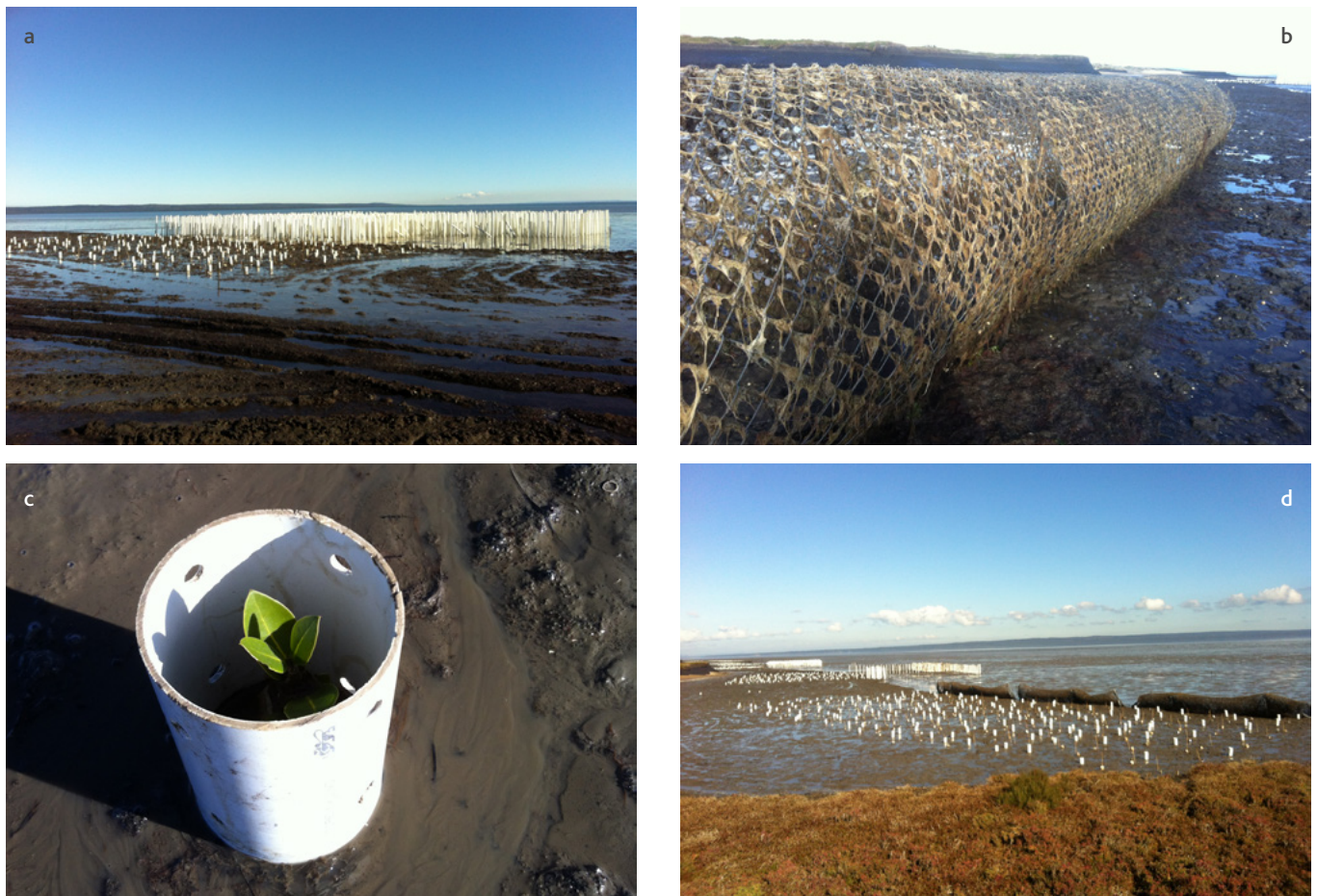
Figure 6.7 Mangrove seedling protective measures; a) PVC pipe pile field; b) wire mesh roll; c) PVC pipe guard; d) experimental setup along Lang Lang coast.
