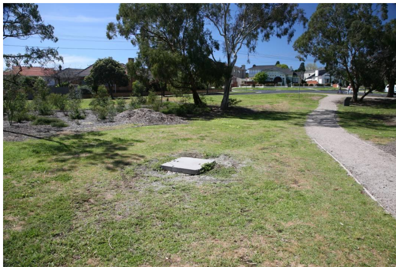
Figure 5 Stormwater Drain junction pit adjacent to soft path in north west of Napier Park
