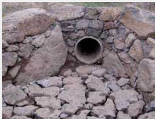
✗ Poor sealing of rockwork.
