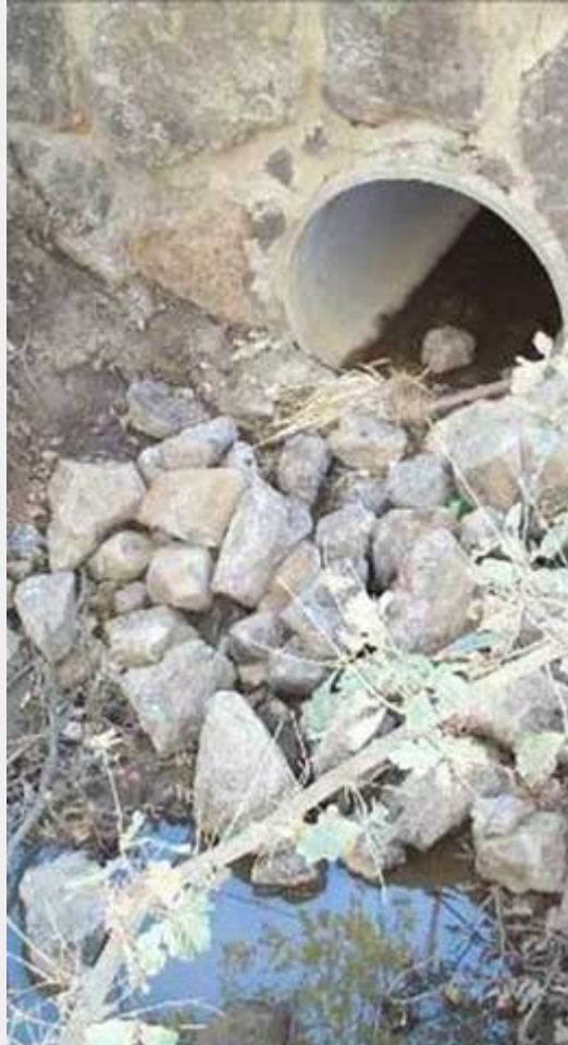
✗ Rocks have simply been dumped in front of outlet pipe - apart from obvious problems with grading, interlocking and sealing of rocks, other problems include rocks projecting above pipe invert, rocks not extended up banks, toe rocks not entrenched into creek bed.
