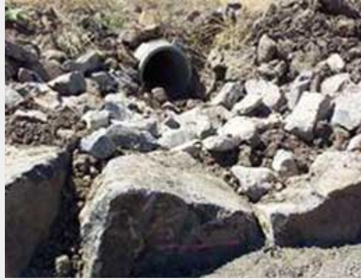
✗ Rocks placed straight on clay without filter/embedment layer.
