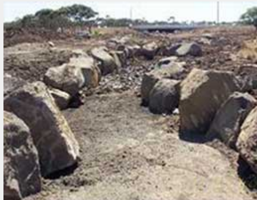
✗ 20mm crushed rock not generally preferred for filter/embedment layer in active waterway.
