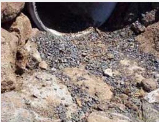
✓ Well interlocked and well sealed rock beaching Refer rockwork in front of pipe.
