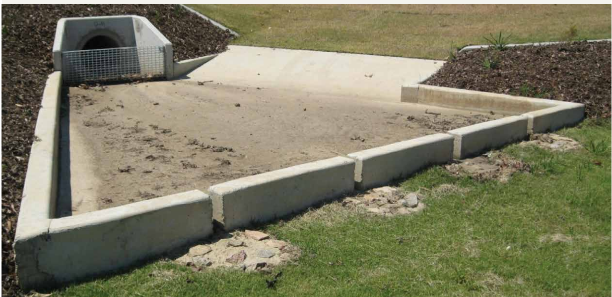
Figure 6 Example of a sediment forebay at the inlet zone of a raingarden (note the raingarden surface is covered with turf to protect the filter media from construction phase sediment loads)
