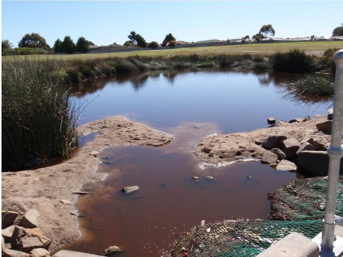
Figure 3: Example sediment pond (Banyan Reserve, Carrum Downs):
