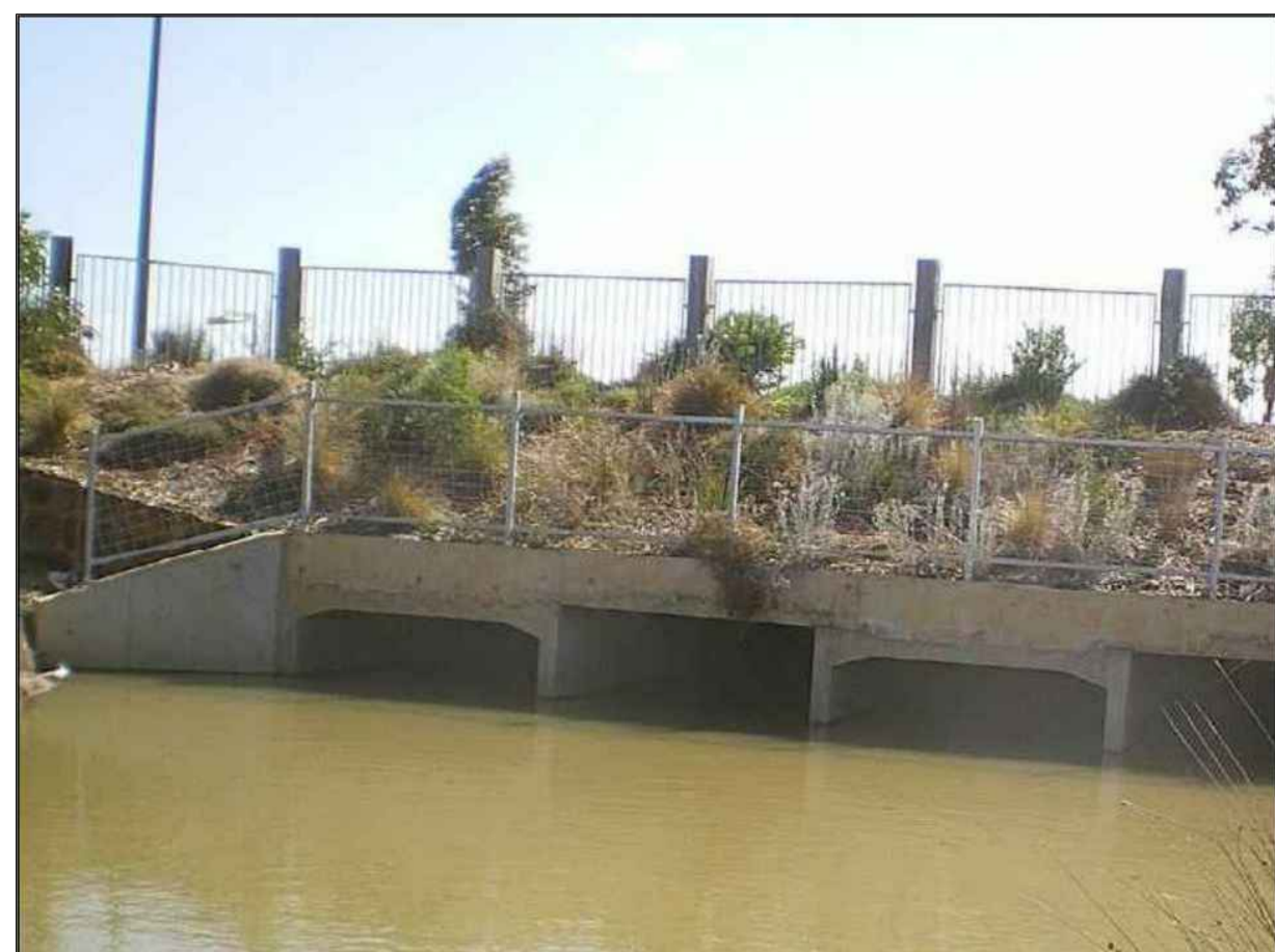
CULVERT MOUNTED SAFETY FENCING PHOTO
