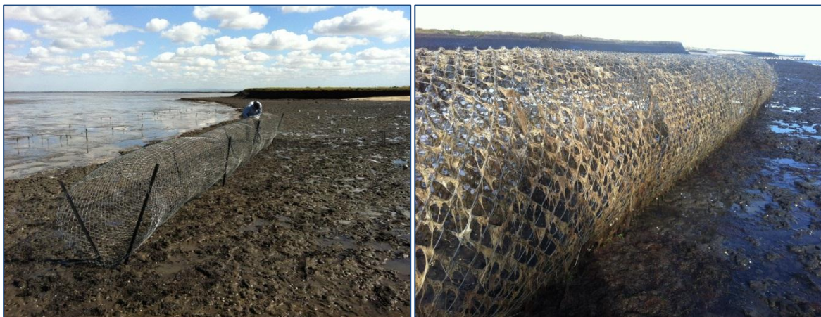
Figure 34: Enviro roll when constructed (left) and 4 months after construction (right) showing significant build-up of algae and other debris.
