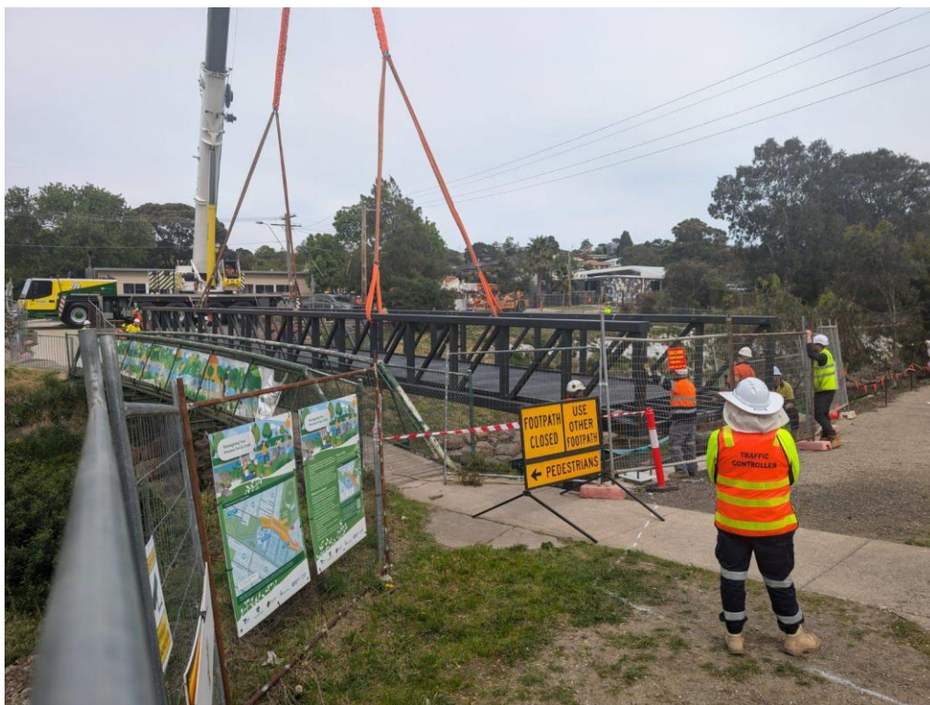
Photo 1 - A photo of the construction site with a crane lifting the bridge into place.
