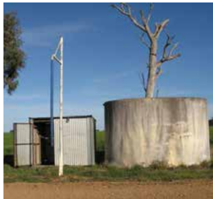
Emergency Water Supply Point, Homebush Road, Wareek © DELWP
