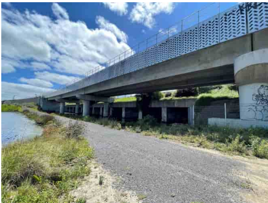
Figure 3-2: Access Track (gravel) downstream of the Footscray Rail culverts (photo taken in 2023).
