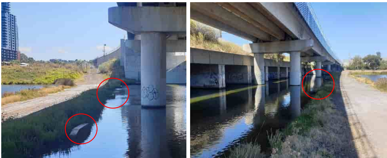
Figure 3-3: Downstream of the Footscray Rail culverts: facing west (left) and east (right). Balancing culverts under the access track circled in red (photos taken in 2023).
