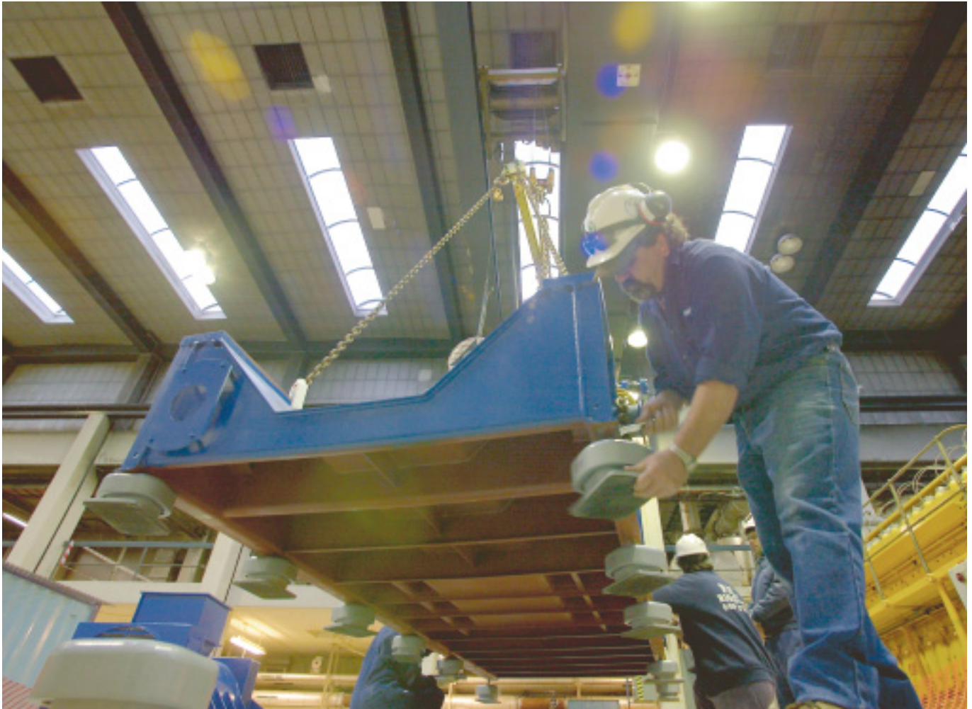
Installing one of seven new generators at the Eastern Treatment Plant, part of the Eastern Green Energy Project.
