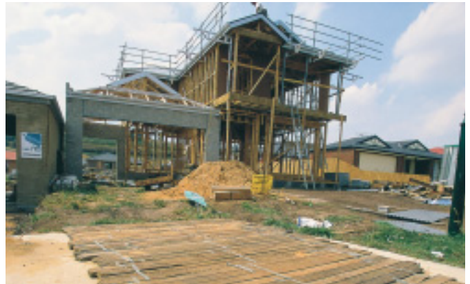
Construction sites are a significant source of stormwater pollution.
