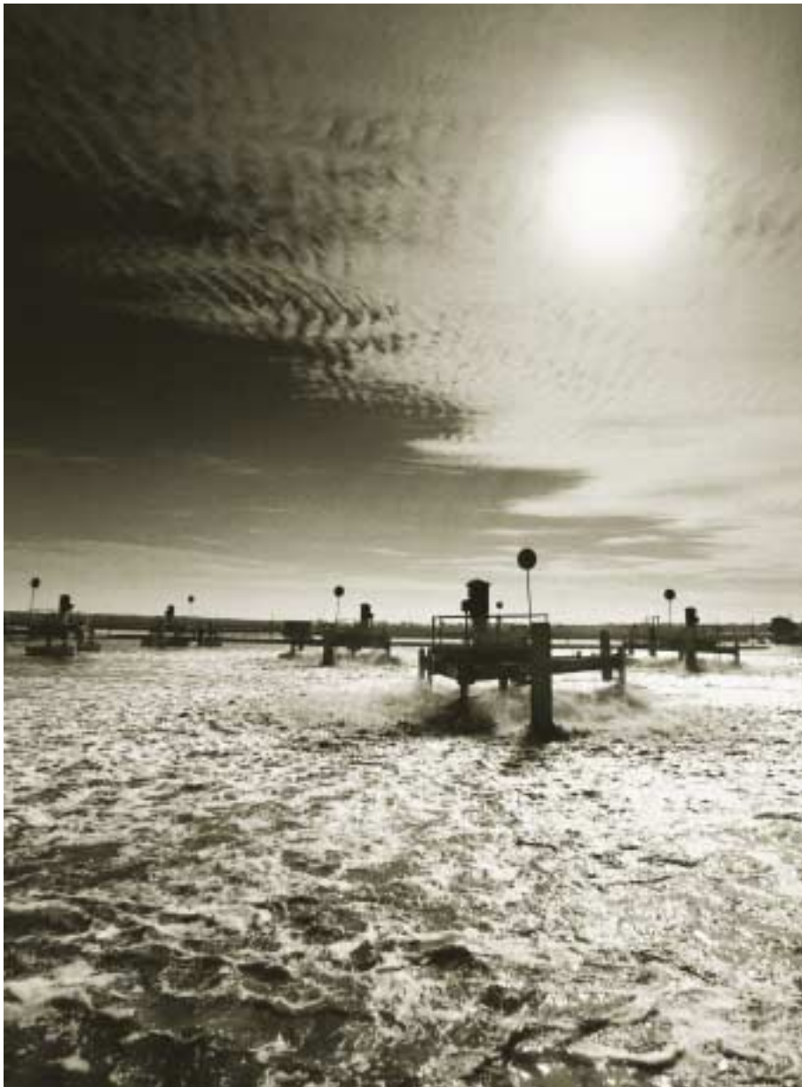
Aerators at work in the lagoon system at our Western Treatment Plant.
