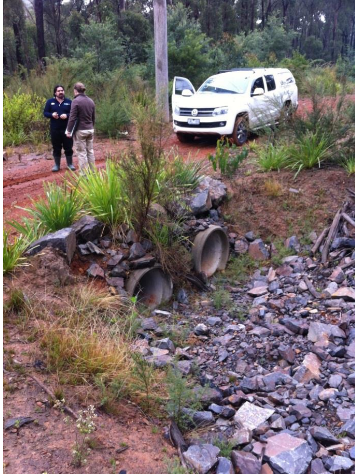
Figure 3. Dual round 'underpass' under the Pipeline Vehicle Maintenance Track, Toolangi State Forest.
